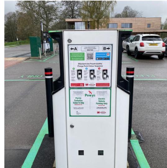
Example of EV Charge point
